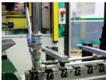
A pair of medium Vortex Tubes cool a solenoid coil after a welding operation.
